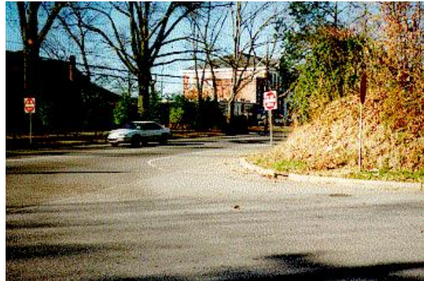
The bank at the corner of Fifth Street Court SE and Second Avenue SE creates a sight distance problem.
