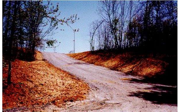
Exit road from the ball fields to Third Avenue Drive SE under construction.
